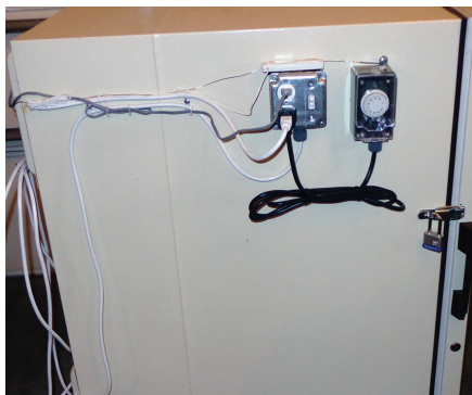
Mounted on the left-hand side of the kiln are the controls, power switch, and outlet, as well as the greenhouse controller. Note the padlock for safety.
